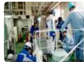
Pump piping line check
